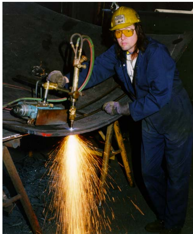
Figure 4.1 An oxygen cutting torch is used to cut the shaped plate to length. After cutting, the slag and metal discoloration will have to be mechanically removed (UG–76).
