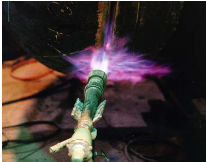
Figure 4.12 A torch is used to preheat this thick walled material prior to making the shell-to-head weld.
