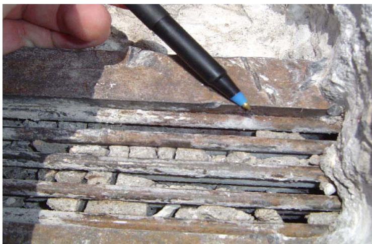
Figure 9. Typical condition of exposed anchorage.
