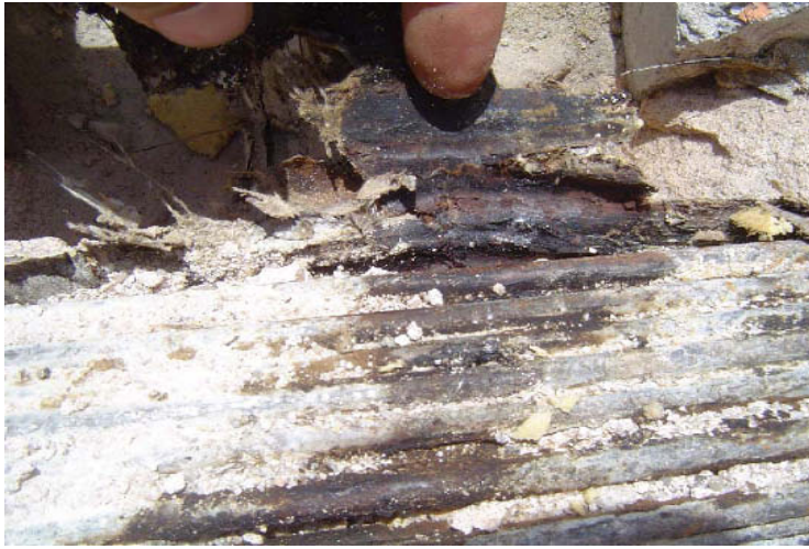
Figure 7. Typical condition of prestressing wires.
