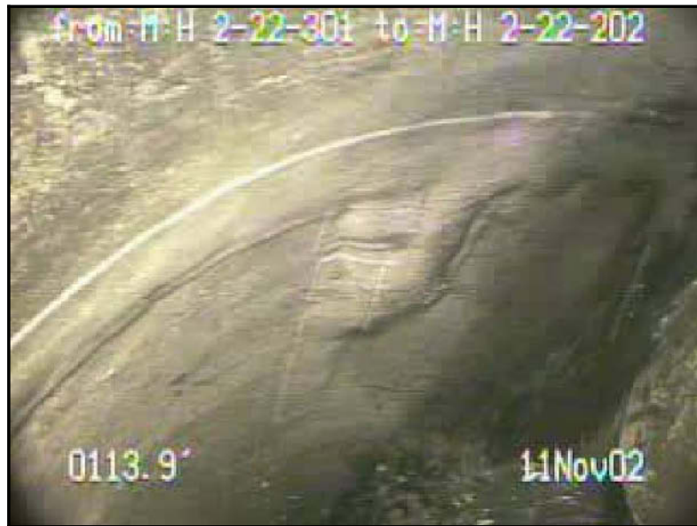
Figure 4. Blister in liner
