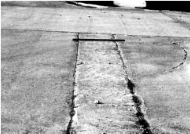
FIG. X2.26 Medium-Severity Patching, Large and Utility Cuts
