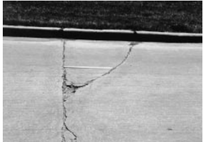
FIG. X2.5 Medium-Severity Corner Break
