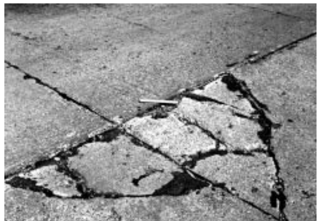
FIG. X2.6 High-Severity Corner Break
