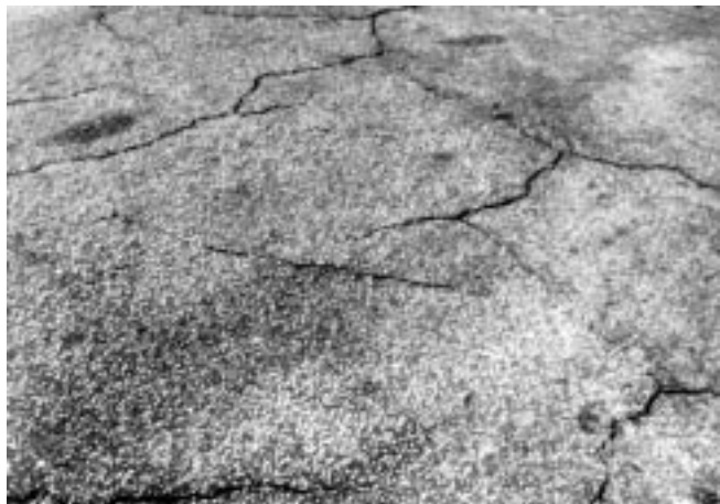
FIG. X1.9 High-Severity Block Cracking
