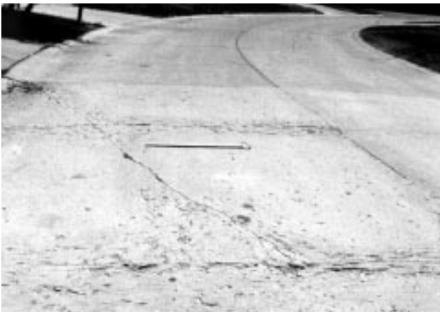
FIG. X2.12 High-Severity Durability Cracking
