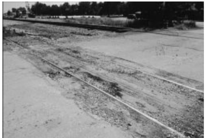
FIG. X1.40 High-Severity Railroad Crossing
