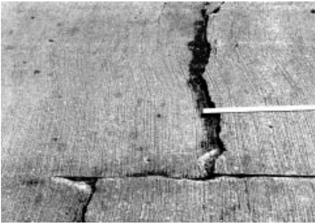
FIG. X2.24 High-Severity Linear Cracking
