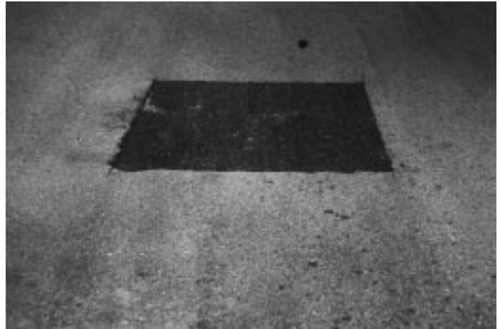
FIG. X1.31 Low-Severity Patching and Utility Cut Patching
