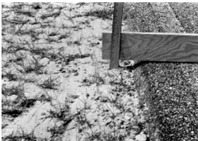
FIG. X1.25 Low-Severity Lane/Shoulder Drop-Off
