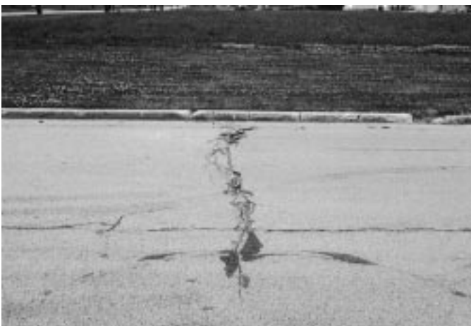
FIG. X1.30 High-Severity Longitudinal and Transverse Cracking
