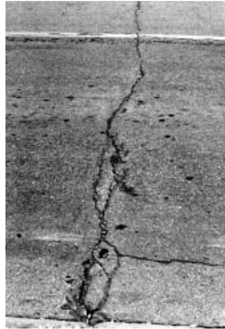
FIG. X1.23 Medium-Severity Joint Reflection Cracking
