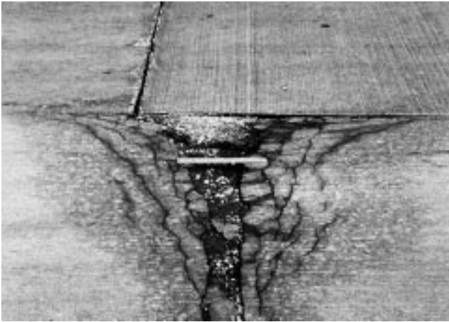
FIG. X2.11 Medium-Severity Durability Cracking
