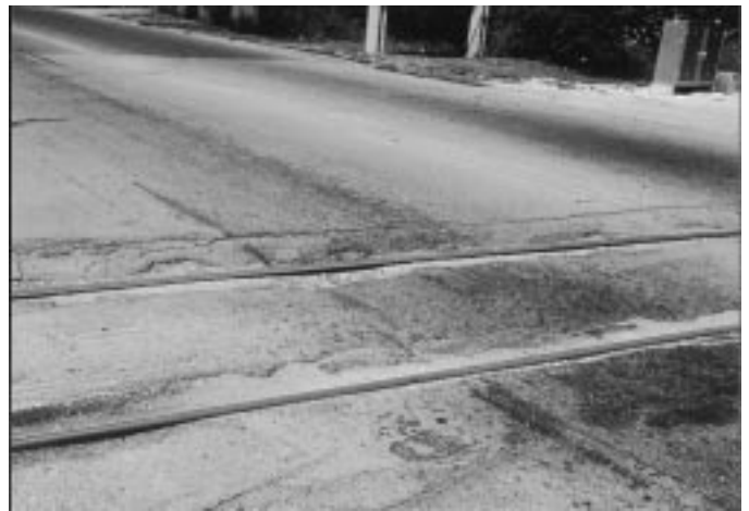
FIG. X1.39 Medium-Severity Railroad Crossing
