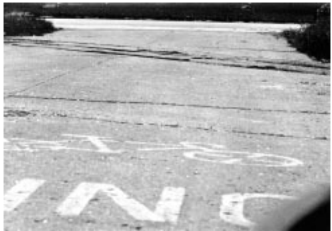
FIG. X2.39 Medium-Severity Railroad Crossing
