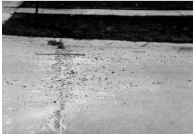
FIG. X2.1 Low Severity Blowup/Buckling
