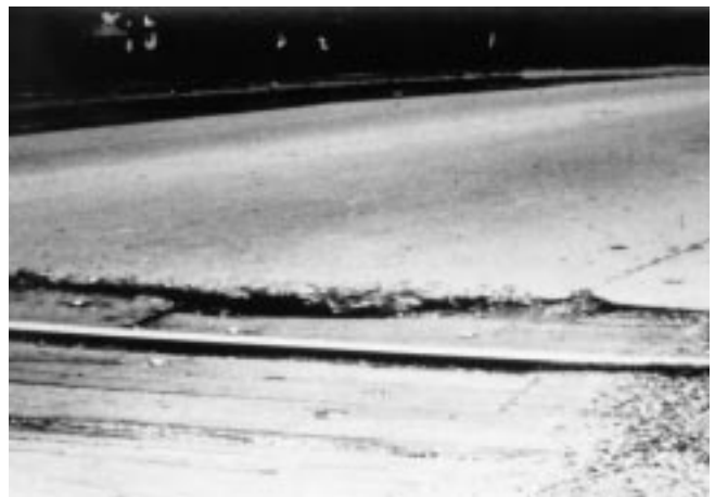
FIG. X2.40 High-Severity Railroad Crossing
