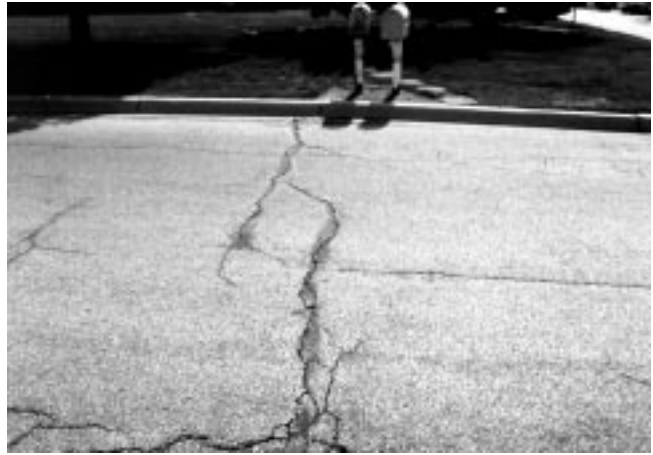
FIG. X1.8 Medium-Severity Block Cracking
