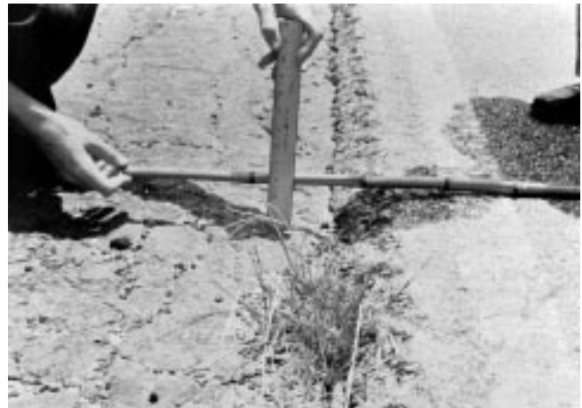
FIG. X1.26 Medium-Severity Lane/Shoulder Drop-Off
