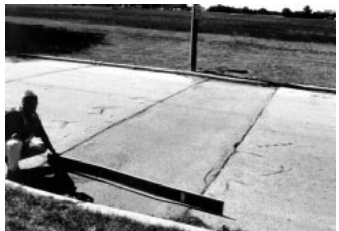
FIG. X1.32 Medium-Severity Patching and Utility Cut Patching
