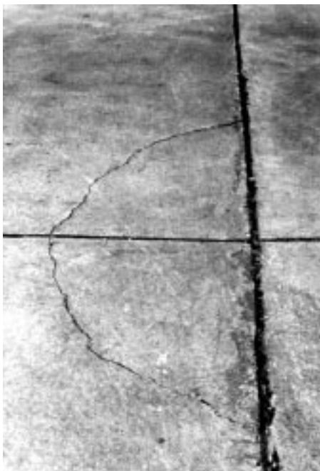
FIG. X2.4 Low-Severity Corner Break
