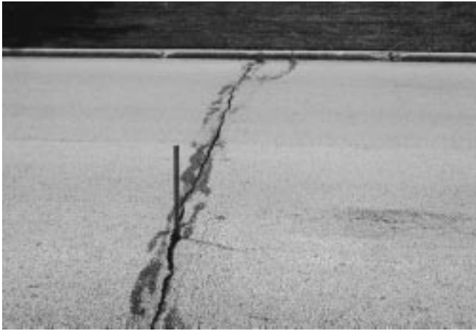
FIG. X1.29 Medium-Severity Longitudinal and Transverse Cracking
