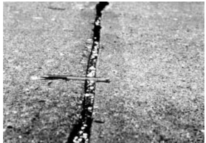
FIG. X2.18 High-Severity Joint Seal Damage
