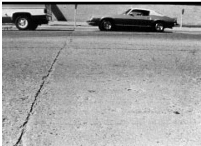
FIG. X2.48 Low-Severity Spalling, Joint
