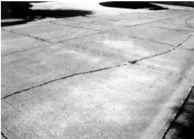
FIG. X2.7 Low-Severity Divided Slab
