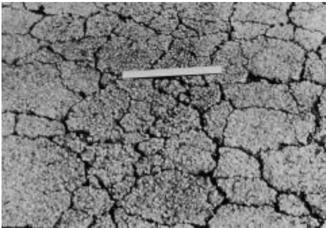
FIG. X1.3 High-Severity Alligator Cracking
