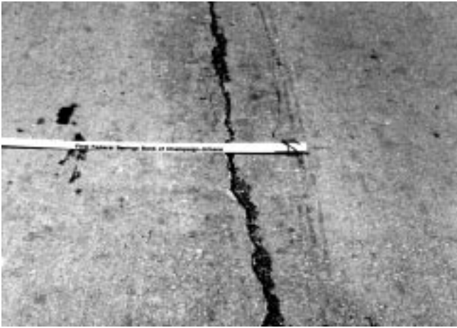
FIG. X2.23 Medium-Severity Linear Cracking
