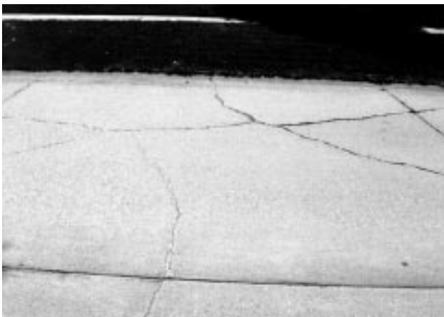
FIG. X2.8 Medium-Severity Divided Slab
