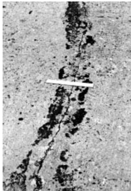
FIG. X2.22 Low-Severity Linear Cracking
