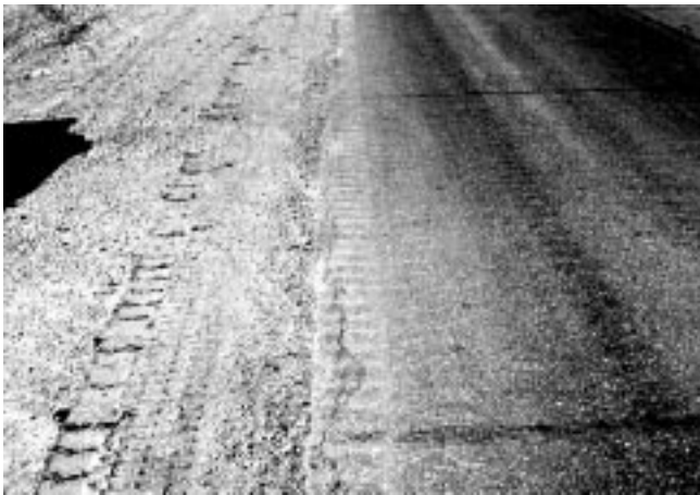
FIG. X1.22 Low-Severity Joint Reflection Cracking
