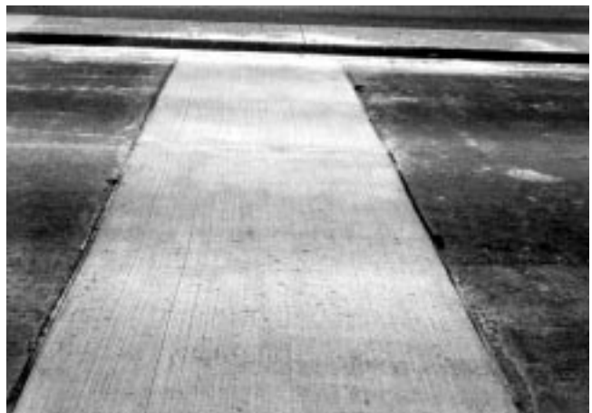
FIG. X2.25 Low-Severity Patching, Large and Utility Cuts
