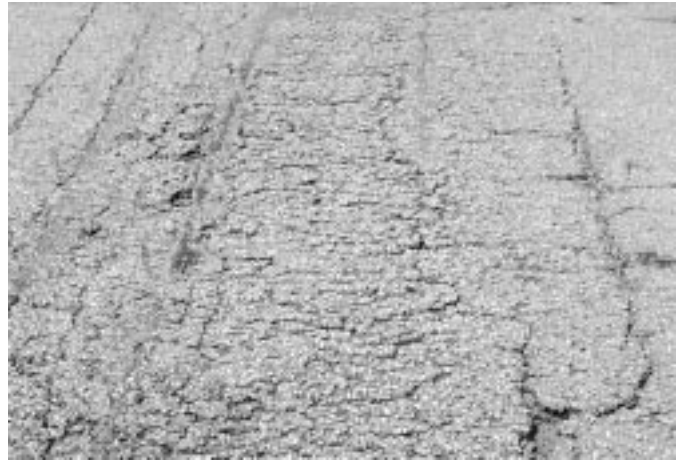
FIG. X1.52 Medium-Severity Weathering and Raveling
