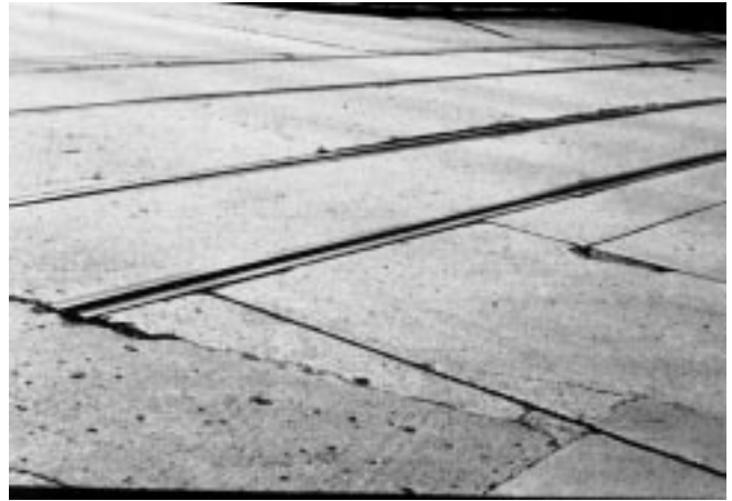
FIG. X2.38 Low-Severity Railroad Crossing
