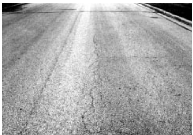
FIG. X1.1 Low-Severity Alligator Cracking
