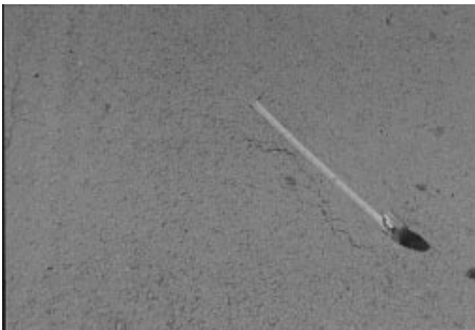
FIG. X1.47 Low-Severity Slippage Cracking
