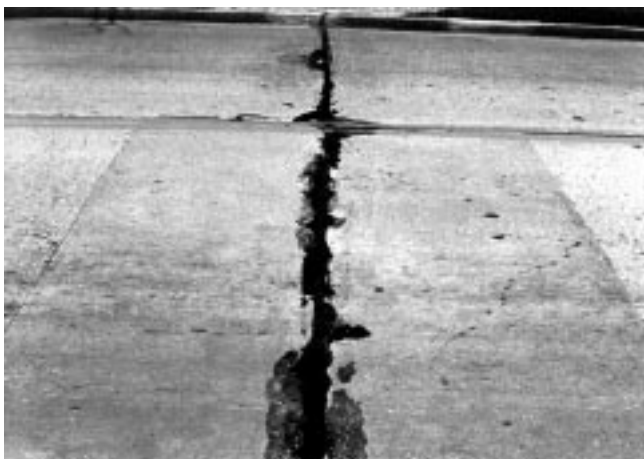
FIG. X2.16 Low-Severity Joint Seal Damage
