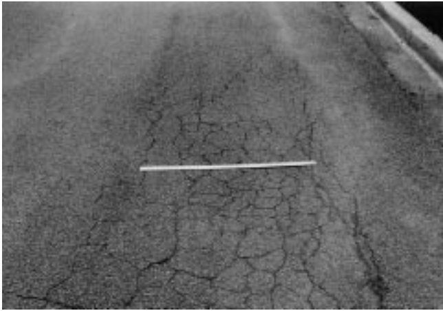
FIG. X1.2 Medium-Severity Alligator Cracking
