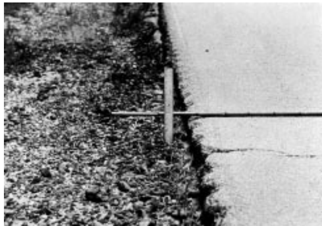
FIG. X1.27 High-Severity Lane/Shoulder Drop-Off
