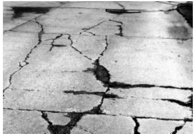
FIG. X2.9 High-Severity Divided Slab
