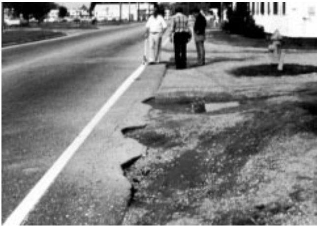
FIG. X1.21 High-Severity Edge Cracking
