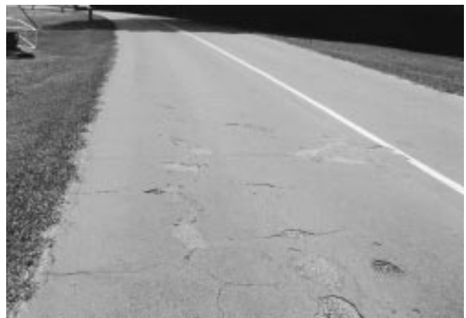
FIG. X1.53 High-Severity Weathering and Raveling
