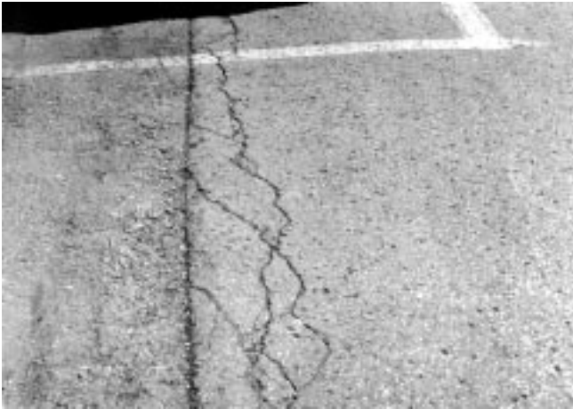
FIG. X1.20 Medium-Severity Edge Cracking
