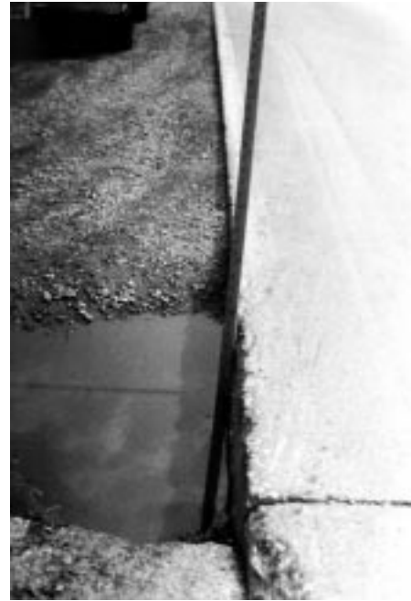
FIG. X2.21 High-Severity Lane/Shoulder Drop-Off
