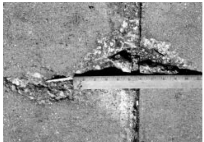
FIG. X2.46 Medium-Severity Spalling, Corner
