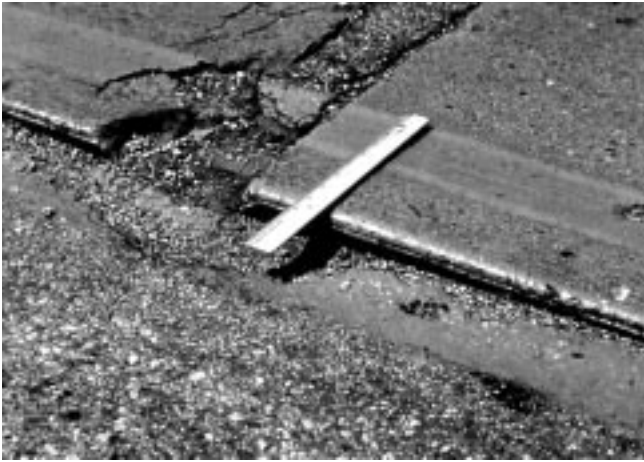
FIG. X2.19 Low-Severity Lane/Shoulder Drop-Off
