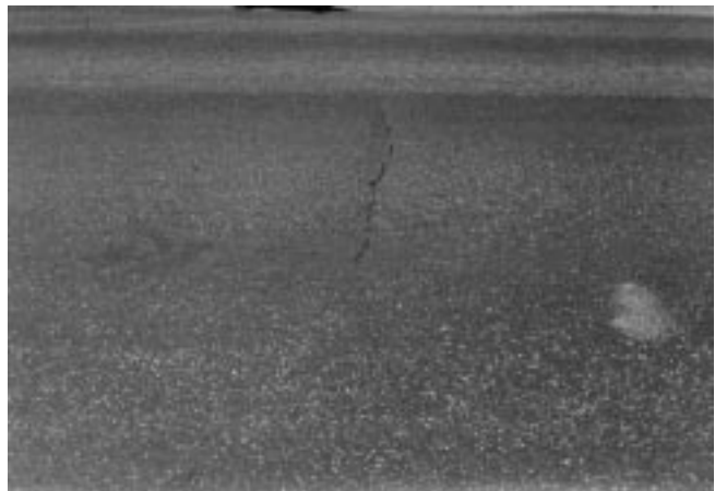
FIG. X1.28 Low-Severity Longitudinal and Transverse Cracking
