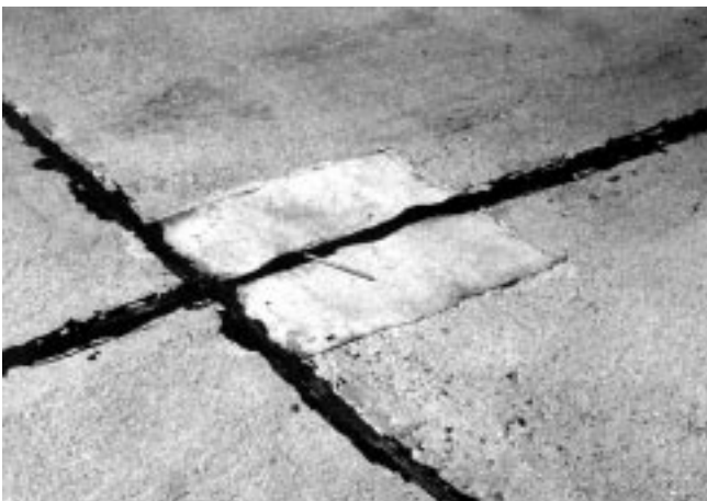
FIG. X2.28 Low-Severity Patching, Small
