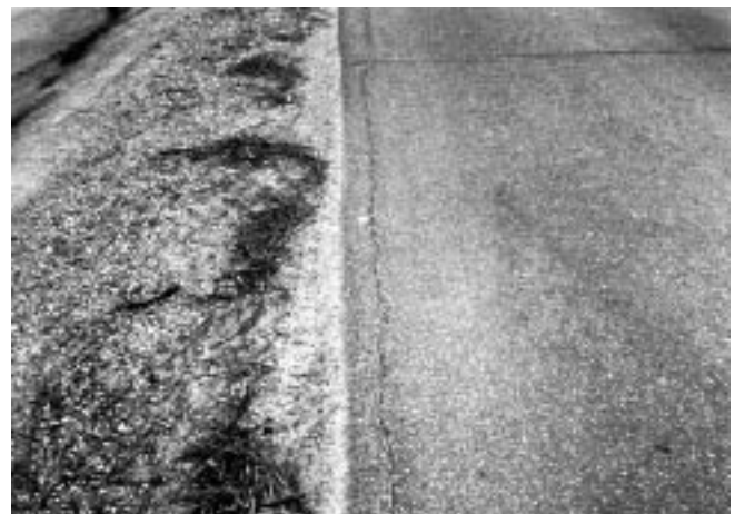
FIG. X1.19 Low-Severity Edge Cracking
