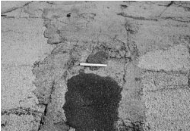
FIG. X1.33 High-Severity Patching and Utility Cut Patching
