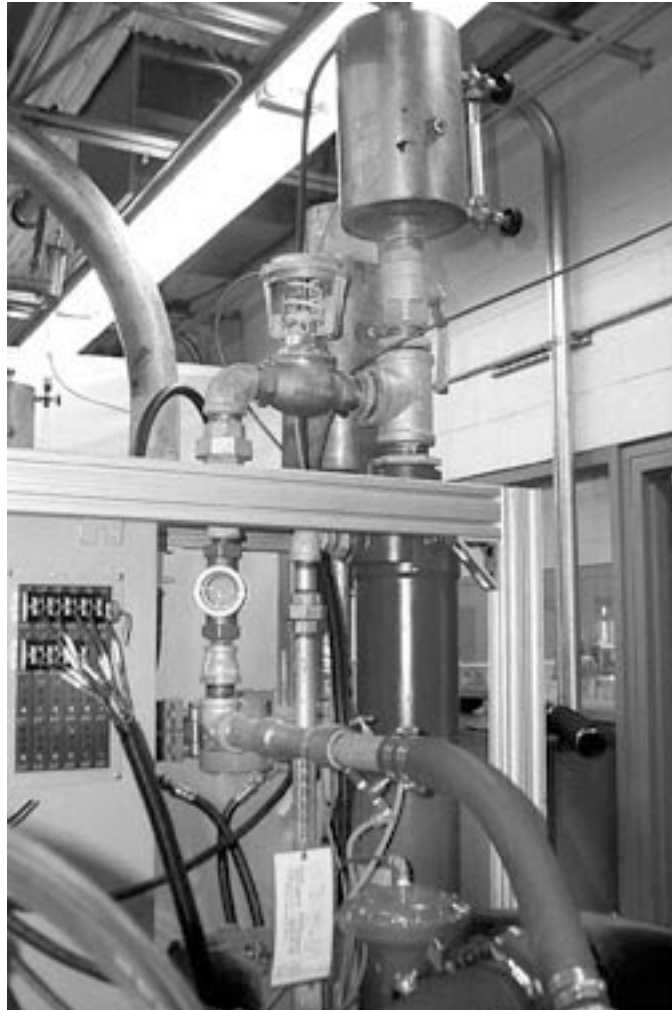
FIG. A3.23 Typical Cooling System, Flow Control Valve, Venturi Flowmeter, Reservoir and Sight Glass
