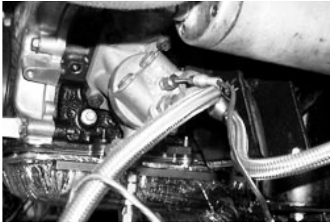
FIG. A3.25 Oil Cooling System, Adapter Housing at the Engine with Typical Fittings for Temperature Sensors, Pressure Tap and Oil Filter
