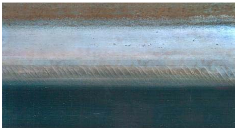
Fig. 10 - Typical example of head-checking on the high rail of a curve
