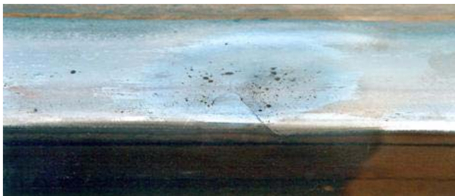
Fig. 14 - Typical V-shaped crack on the running surface
