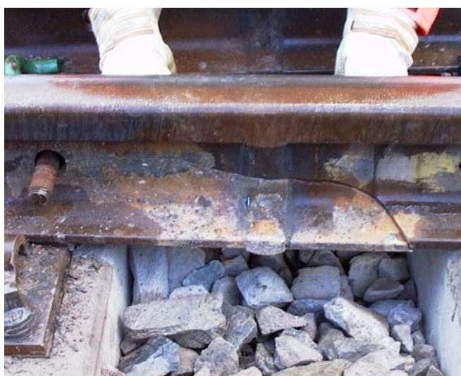
Fig. 3 - Typical example of a horizontal crack on an aluminothermic weld
