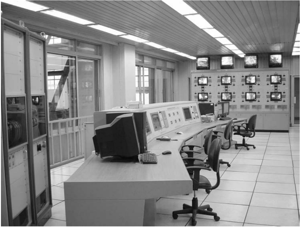
FIGURE 14.7 The control room.
