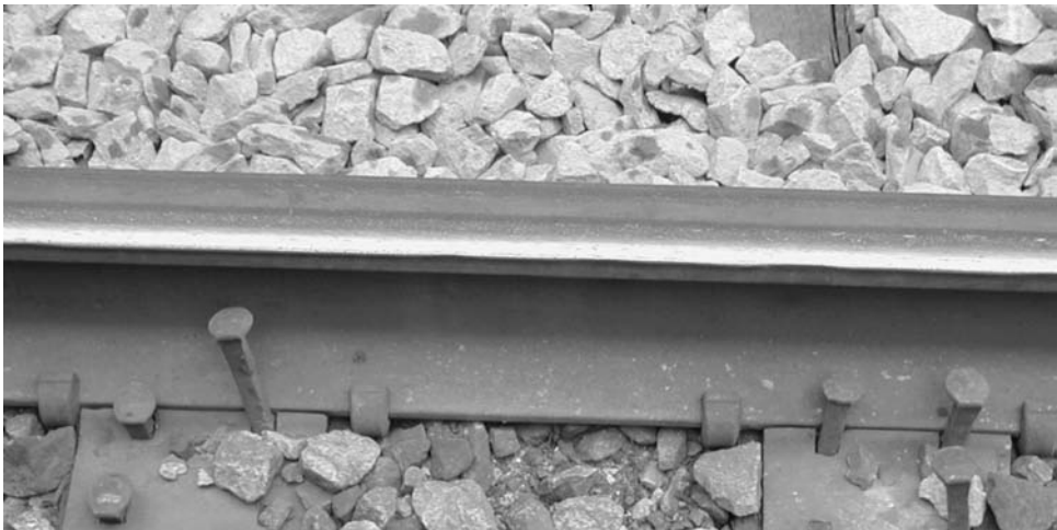
FIGURE 8.25 An example of loose fasteners.
